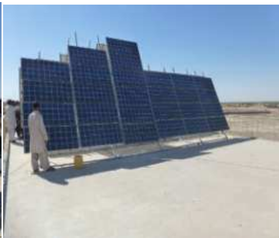
Solar panels (West side)
